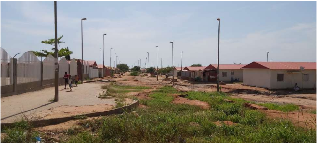
FIGURE 77 ERODED DIRT ROAD IN A PANGUILA NEIGHBORHOOD
